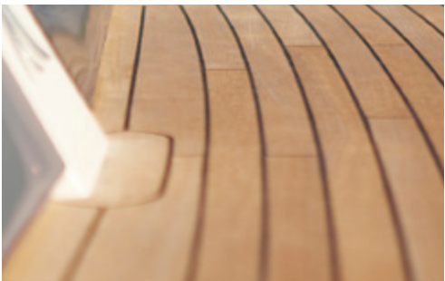
Teak on side decks
