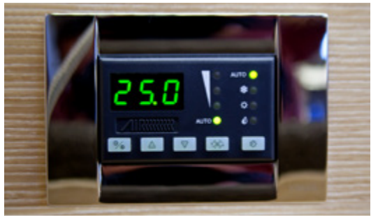
Air condition (12.000 BTU) with 1 outlets
